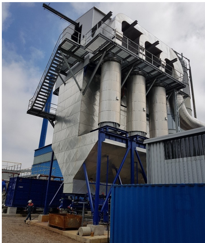
Figure 4. Three AHEX modules installed at TRIMET Hamburg [6].
