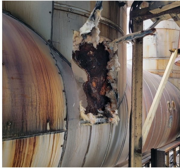
Figure 1. Example of corrosion under insulation.
